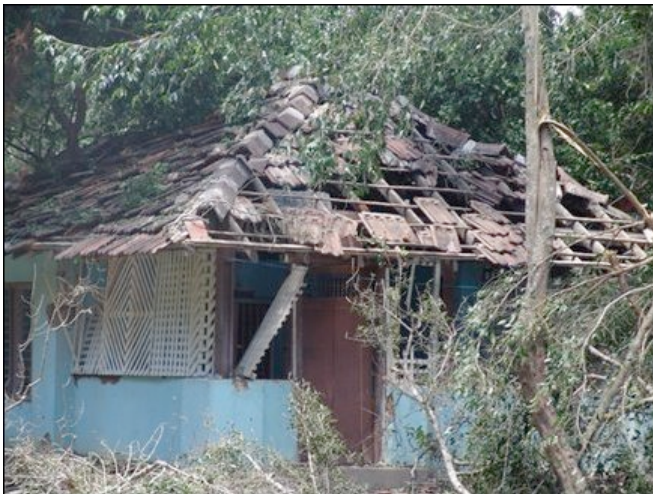
A building of Sencholai, destroyed in SLAF bombing Sencholai attack "pre-meditated, deliberate and vicious"- TNA
