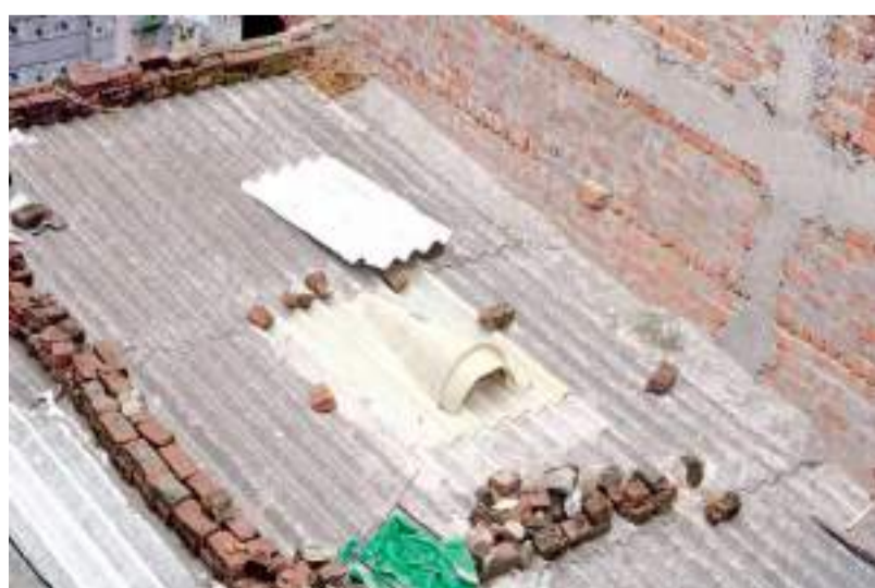
An 'Air-Lite Ventilation' roof facilitated by Mahila Housing Trust at Surekhaben Patil's home in Ahmedabad. Mahila Housing Trust has enabled the installation of more than 200 of this type of roof.
